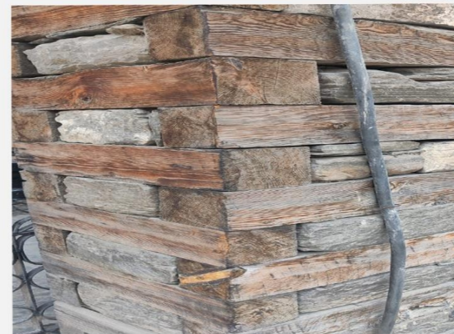
Layering and interlocking timber and stones in the walls provides strength, stability and flexibility.
