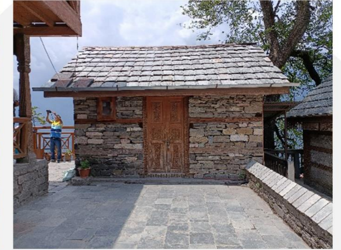
Stone slates were used for pitched roofs that are used to avoid the collection of snow.
