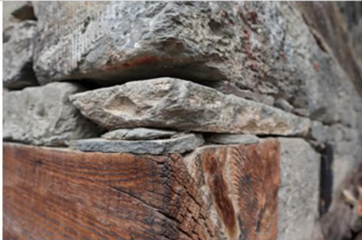
For the better fixing of wood and stone, small chip stone is placed in between of two courses.
